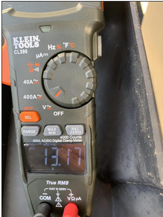
Battery while Charging
