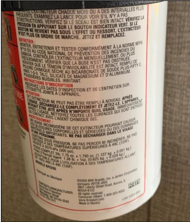
Extinguisher inside front door
