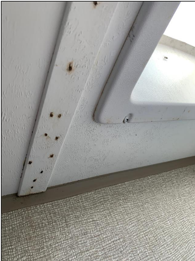
Above the shower on ceiling
