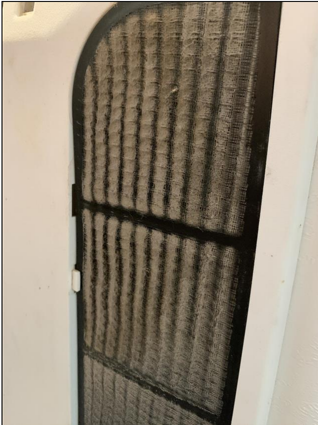
Air Condition filter
