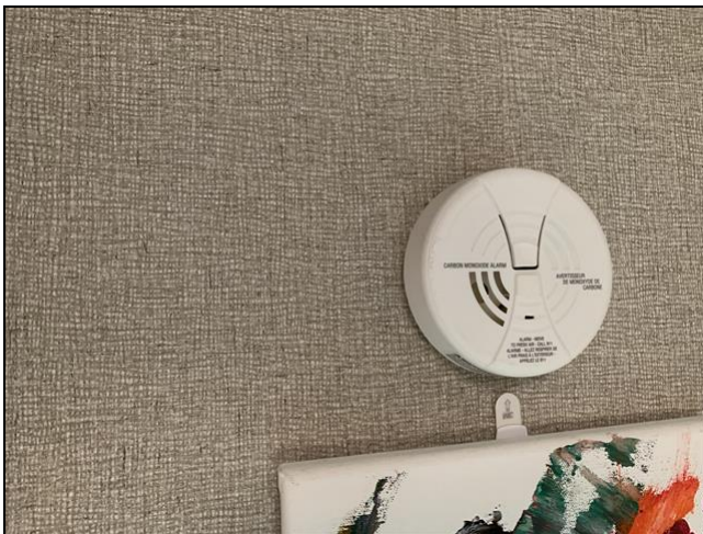
Carbon Monoxide Detector located in front bedroom
