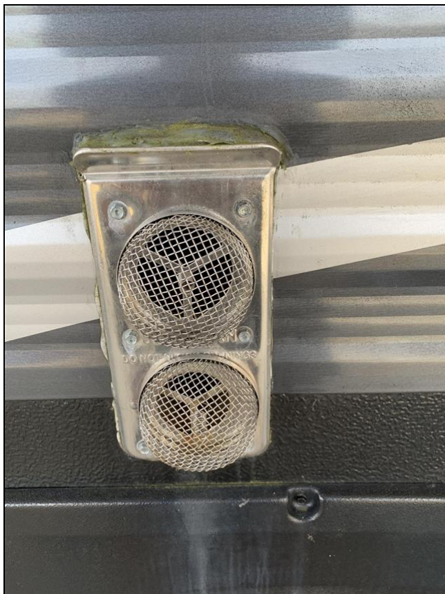
Furnace intake and exhaust
